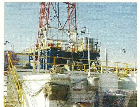
克拉玛依油田防爆照明 Explosion-proof Lighting Fixture in Karamay Oil Field
